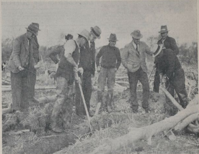
A TE ANAU'S PROBLEM.—Yesterday afternoon members of the Te Anau branch committee with the newly Engineer Mr. B. Grant inspected the work being done to reconstruct the throat of a tunnel from the Transvaal power.
