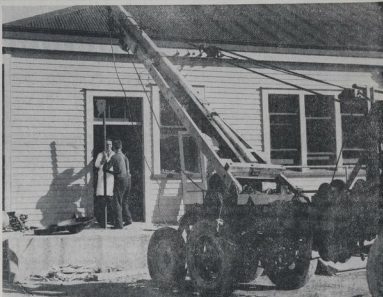
NEW EQUIPMENT FOR SHIPPER HOSPITAL —A large hoisting-machine is to be placed in position by the use of this large beam. On 2. A hoist is now supererecting the work.
