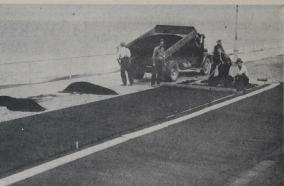
IMPROVEMENTS TO THE MARINE PRAISE.—Landing along a concrete surface on the new playing arena at the recreation grounds of the Heralds Parade, Napier. These arena will be used as tennis courts in the summer and basketball courts in the winter.
