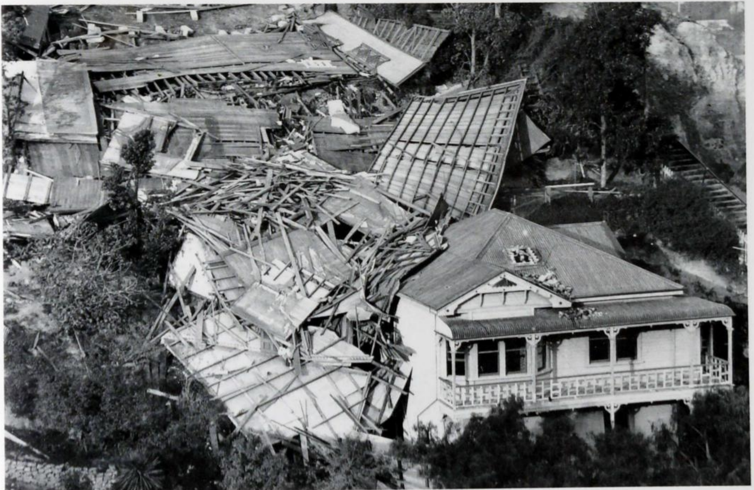
Wooden houses were rarely damaged severely, but this was an exception, jumping off its piles and cascading down the hillside. Its site, above Faraday Street, is still vacant.
