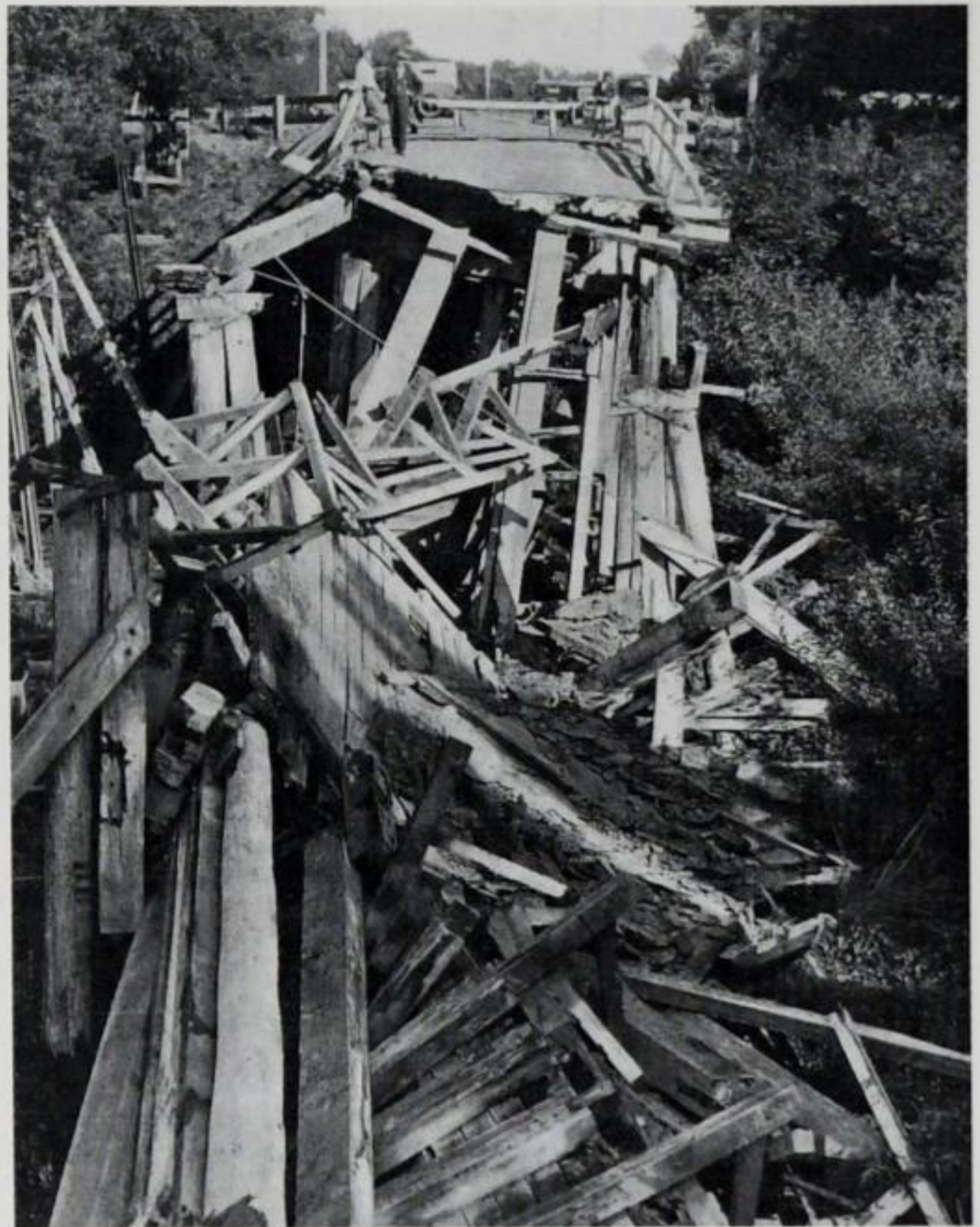
The bridge on the Hastings - Havelock North Road collapsed, bringing down a water main..
