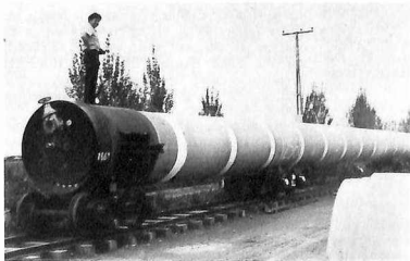
LEFT: Part of a string of sewer pipes mounted on ex-NZR bogies on a track laid along Richmond Road, Clive, ready for launching as part of the Hastings City Council's submarine sewer outfall project, photographed in 1980.
