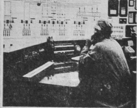
SOPHISTICATED CONTROL systems are an integral part of the Hawke's Bay Electric Power Board's organisation. Shown here is the nerve centre, the operations control room in Hastings.
